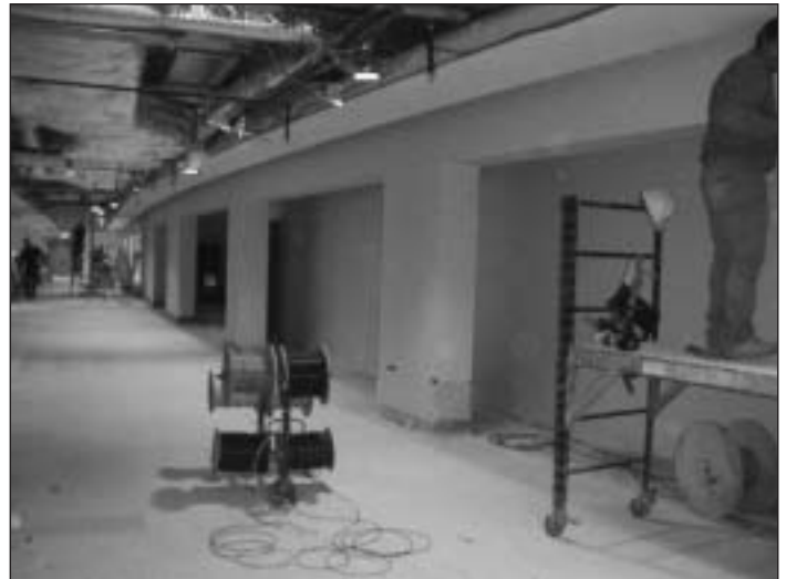
Hallway leading from the Shock Trauma waiting area to new cafeteria and where the new Subway and other vendors will be located.
